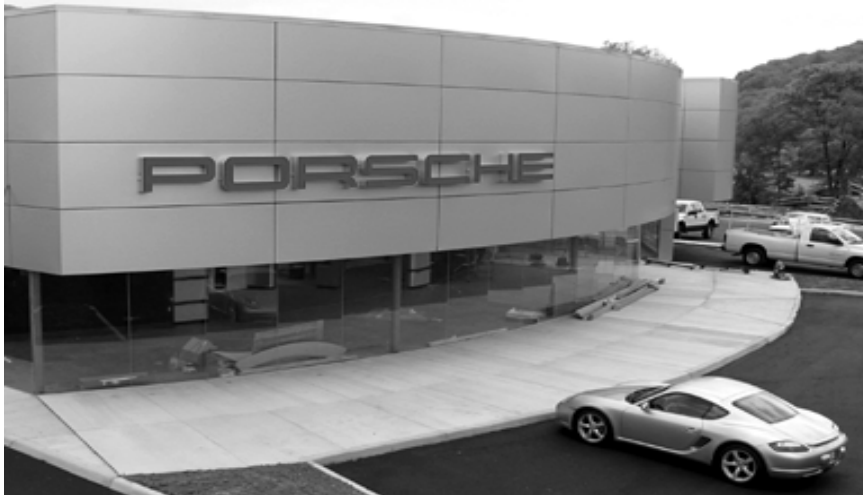
Construction nears completion at the new Hammersley Auto Group Porsche dealership in Roanoke.
